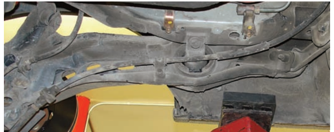
The original brake cable was removed from the car by disconnecting the brackets that secure it to the body pan.
