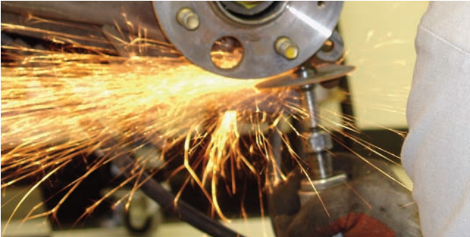
Using a three-inch cut-off wheel the small protrusion was removed as seen here.
